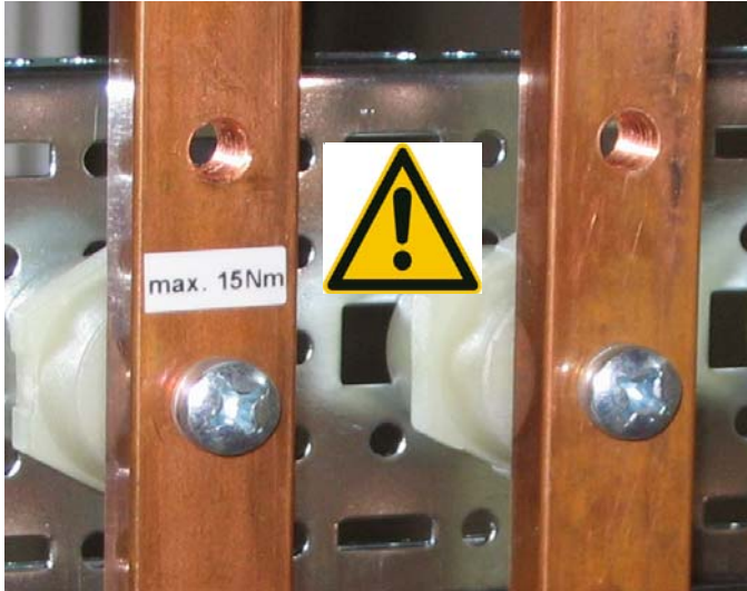
Max. torque for cable lugs on the copper rails 15 nm
